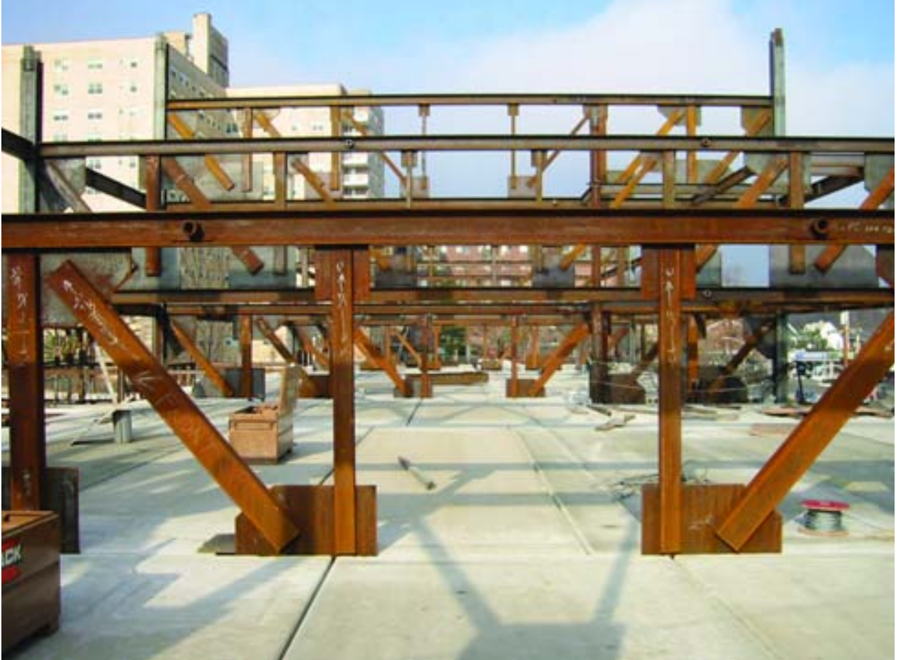
By concealing the trusses within permanent partitions, staggered-truss framing provides large, flexible open spaces.
