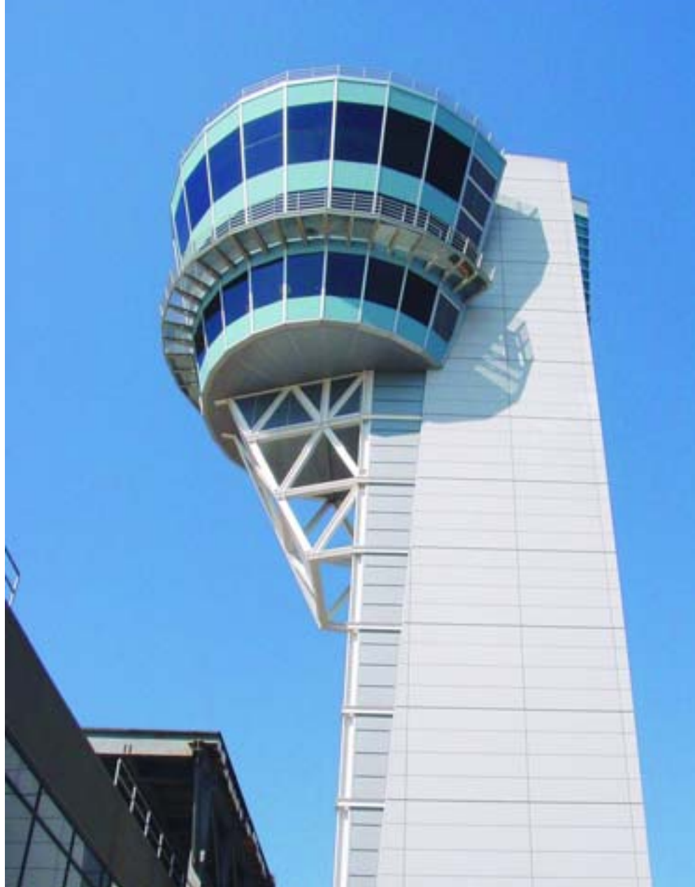
An intumescent coating protects the cantilever truss members against corrosion and fire while providing a smooth appearance.
