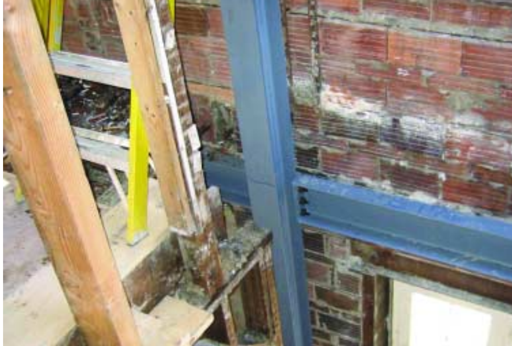
Steel framing was inserted into the existing structure prior to the demolition of the existing wood framing.
