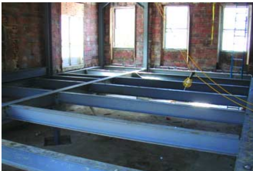
Steel floor framing for the new gymnasium before installation of the non-composite metal deck and concrete floor.
