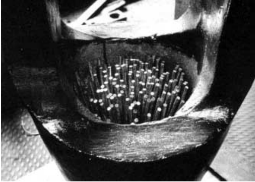
Broomed cable at cable and socket joint. Image from page 11, Harris James, Pui-K Li, Masted Structures in Architecture , Butterworth Architecture, 1996.
