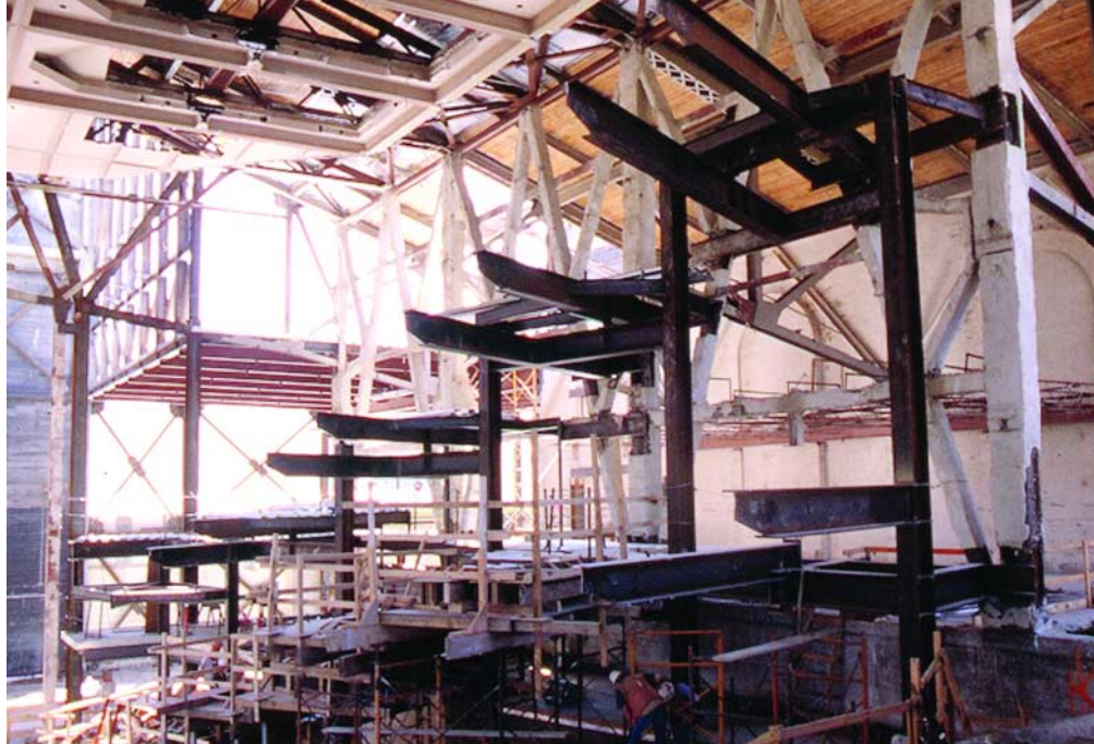
Five new balconies framed with structural steel cantilevers were added on each side of the auditorium. Photo courtesy Michael Dickter and Magnusson Klemencic Associates.
