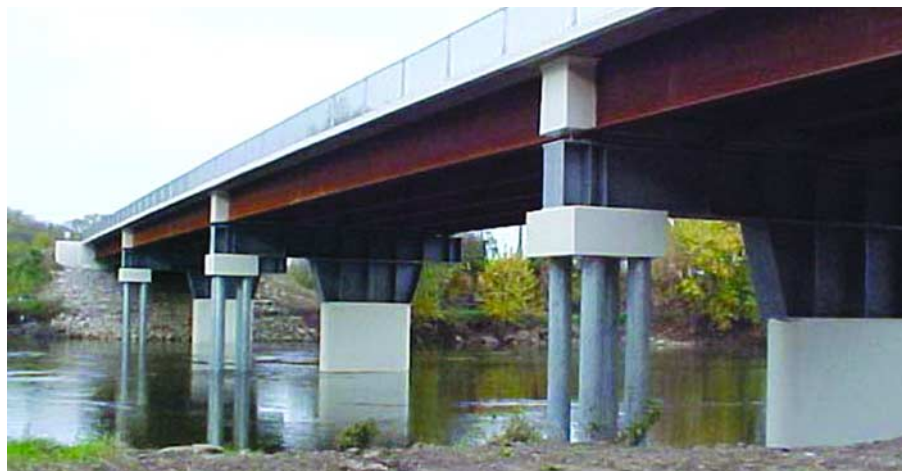
The structure was widened by 10' on the south side. The additional width was supported by new piles in groups of four.
