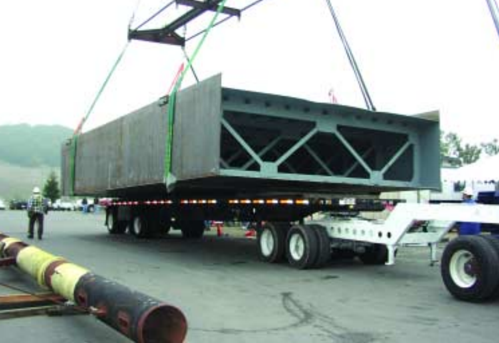
A 180-ton crane moved sections of the ramp around the fabrication yard.
