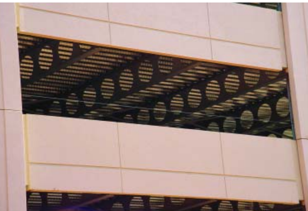
The exterior design of the new five-story parking deck for Lowe's Companies, Inc., was designed to unobtrusively blend in with its natural surroundings.
