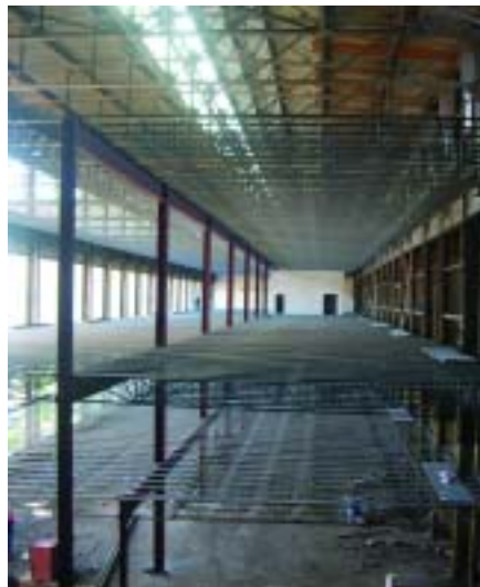
New steel framing added multiple levels of office space to the tall bays. Two of the buildings used wide-flange beams and the third building (shown) used steel joists.
