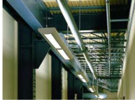
Haunches fabricated from steel plate were welded to the existing steel columns to support the re-used (and repositioned) crane rails.
