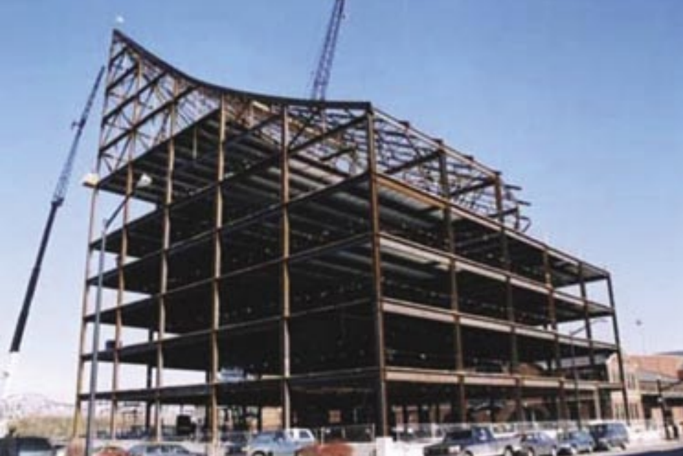
The roof is framed with steel trusses along radial lines with 2" HSS members as purlins.
