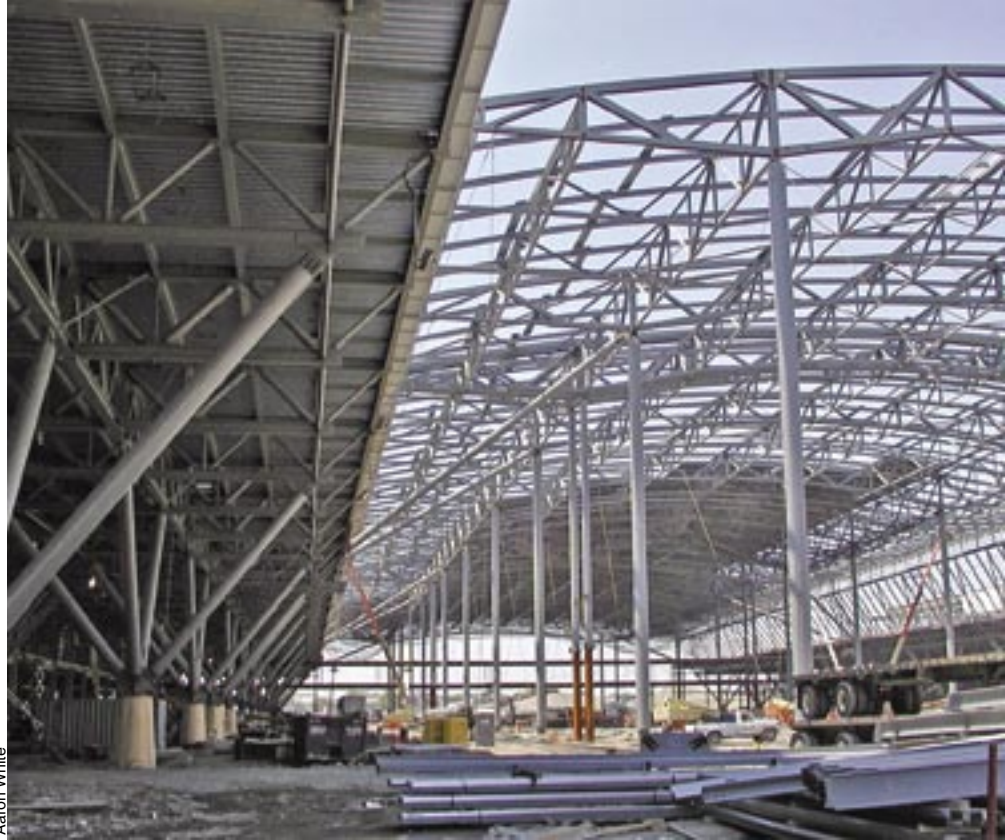
80'-tall pipe columns support the 300'-wide high roof, while its lateral stability is provided through bracing down to the low roof at only four locations between expansion joints. Low roof V-columns provide both gravity support and lateral stability to the entire exhibit hall roof while maximizing useable exhibit hall floor space.
