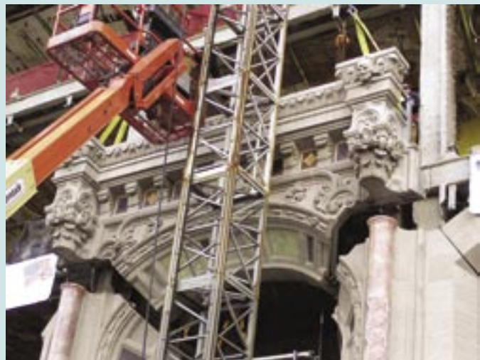
The restored center panel of the grand arch is lowered into place above the main entrance. This panel weighed over 20,000 lb.
