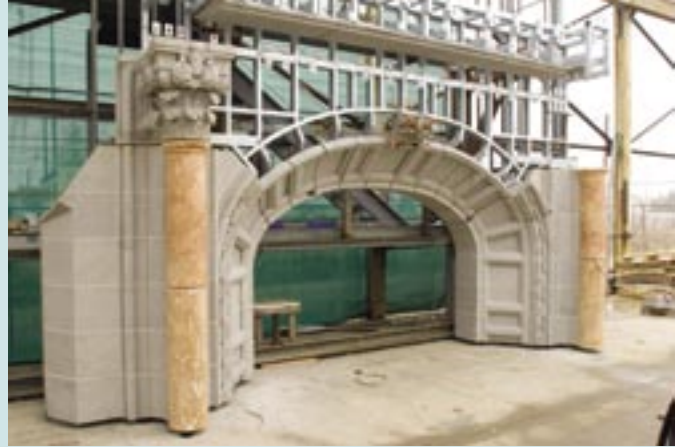
The damaged grand arch at the main entrance (shown on previous page) was reconstructed using original and new stones attached to steel truss panels. Note that the center of the arch is part of the unfinished section.
