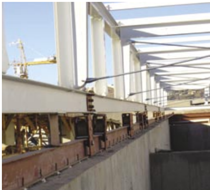
Parallel steel rails support the 38 sets of wheels attached to the movable steel structure.
