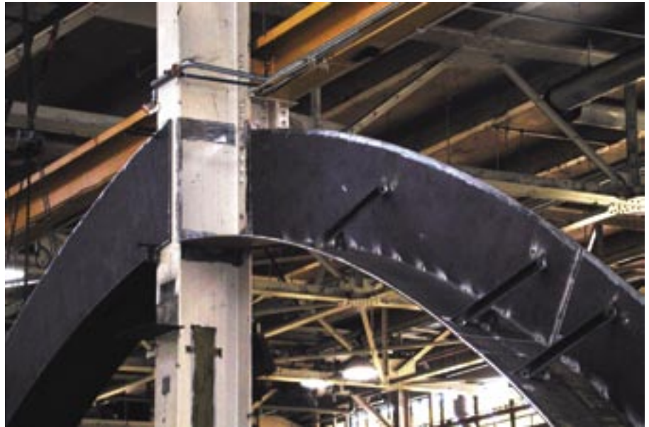
At the crown of the arch, the top and bottom flange plates were extended into and between the flanges of the W21 column.
