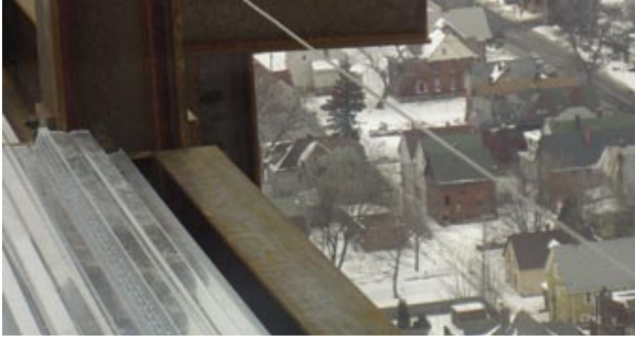
Perimeter beams and girders were connected to the exterior flanges of perimeter columns to minimize the slab pour-stop cantilever.
