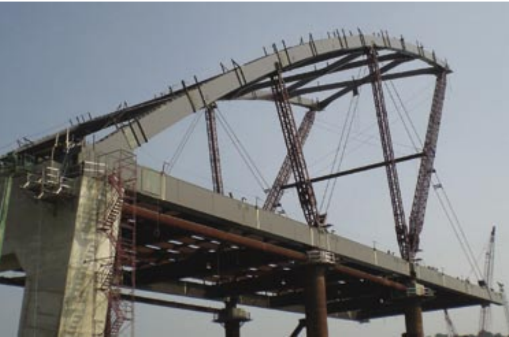
The west arch was set in place off of Pier 3 in July 2006.
