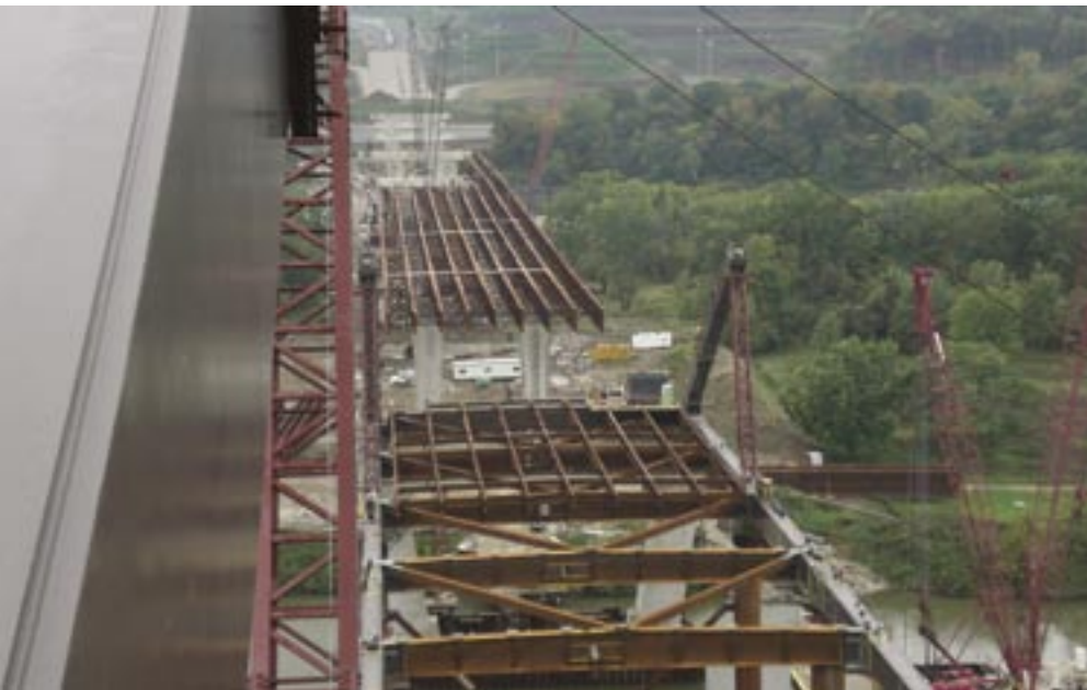
The use of high-performance structural steel allows the Blennerhassett Bridge to be constructed with fewer piers.
