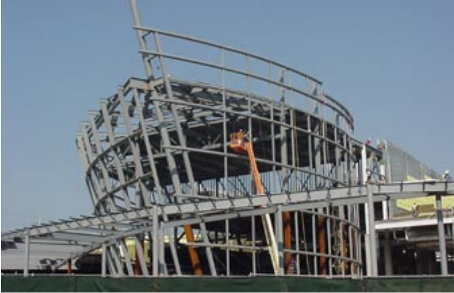
Erection of the bow of the “ship” supported by a 24-in.-round HSS leaning at approximately 15°.
