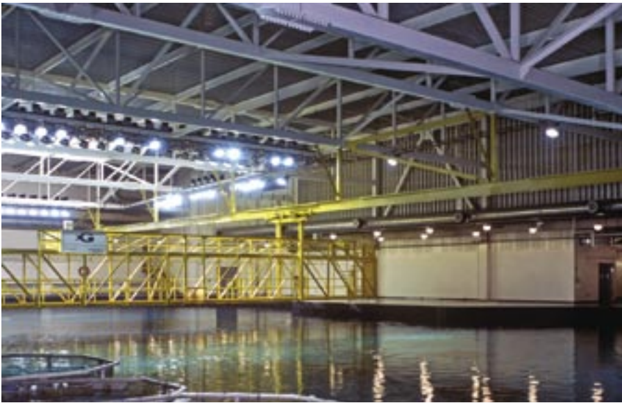
Roof trusses and gantry over the Ocean Voyager exhibit, a saltwater tank measuring over 260 ft long, 120 ft wide, and 30 ft deep at its deepest point.
