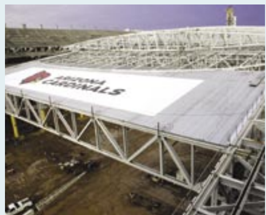
Chicago Metal Rolled Products curved 402 tons of 12" square tubing for the retractable roof of Phoenix Stadium in Glendale, Arizona.
