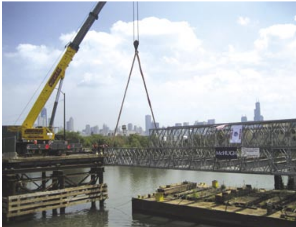
The center section of the temporary North Avenue bridge is lifted into place. Photo by Chicago Department of Transportation.
