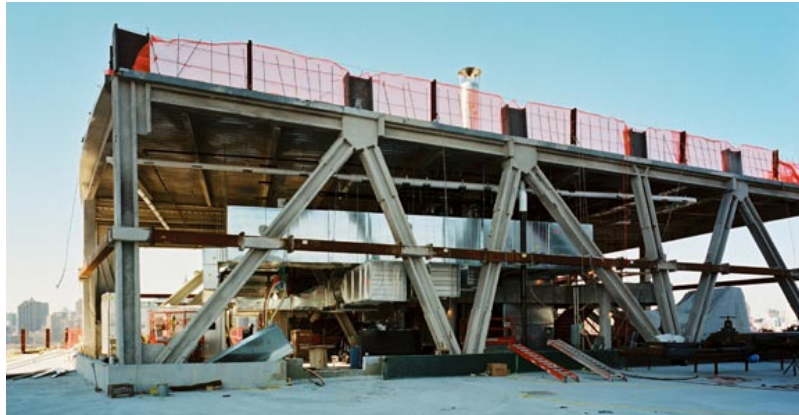
Below: Transfer trusses transition the columns from the future office tower to the columns of the podium structure.
