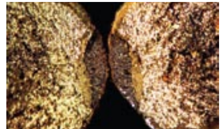
Close-up view of cable corrosion on the Forth Road Bridge.
