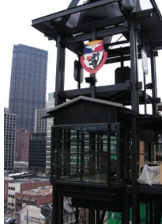
Right: The tower columns support the pedestrian bridge; access to the bridge occurs through the adjacent structures.
