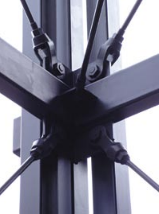
Steel rods and clevises provide visually unobtrusive lateral bracing for the supporting towers.
