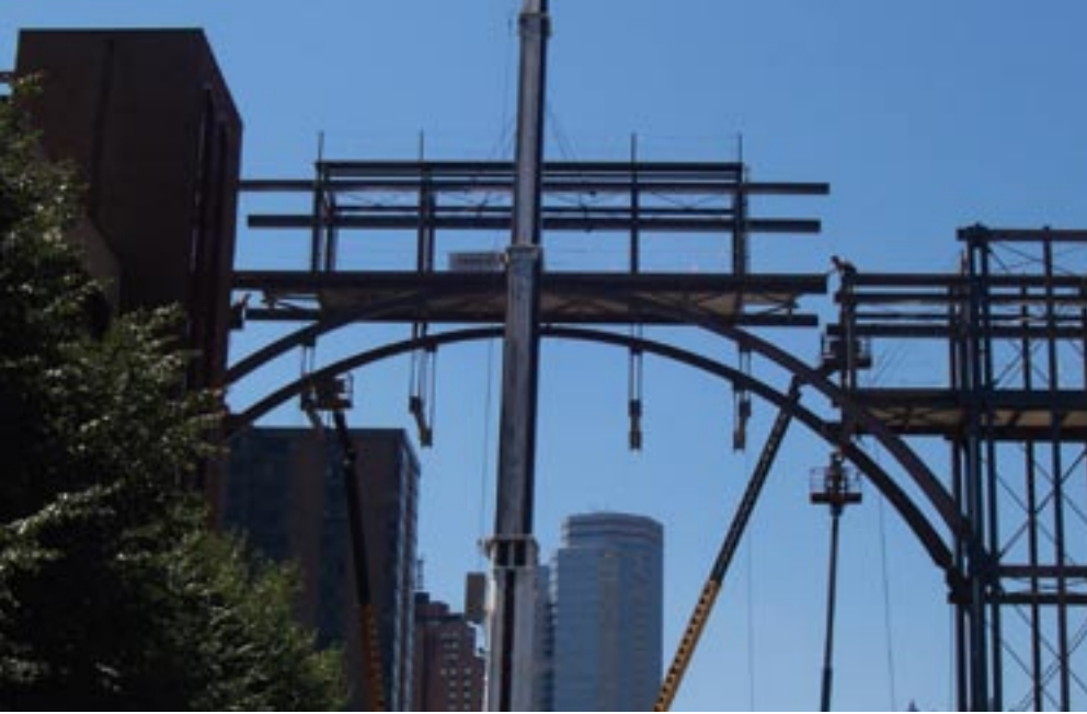
Above: One inch was allowed for tolerances when erecting the prefabricated center span.
