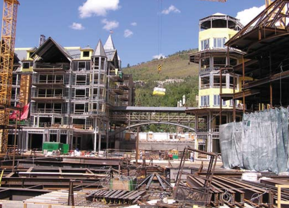
An 85-ft pedestrian bridge connects the east and west areas of the Arrabelle development. The entire project had more than 500 steel beam penetrations.
