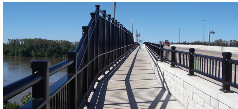
Ornamental pedestrian fence and handrails made from hollow structural sections adorn the new Christopher S. Bond Bridge.
