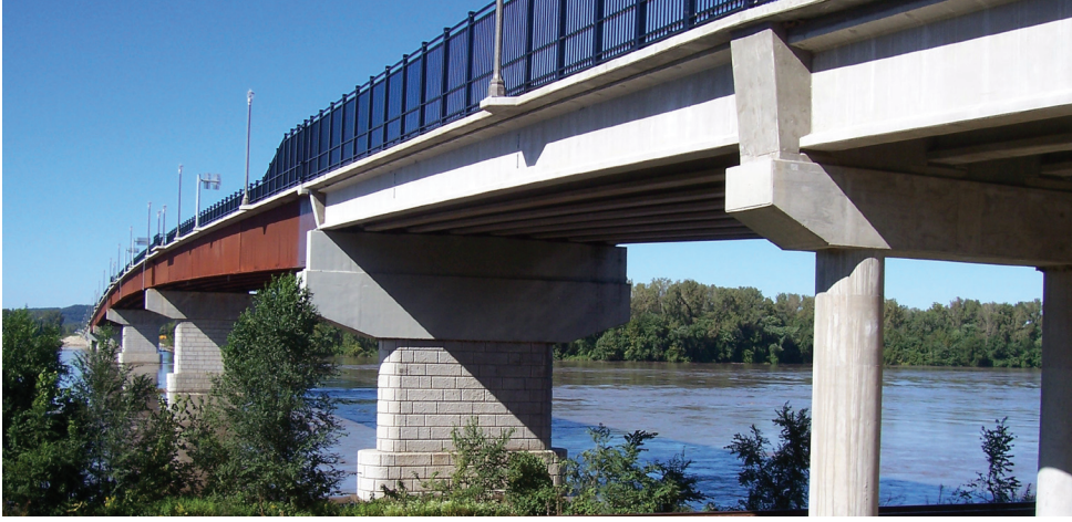
High-performance steel was used for the negative moment flange plates over the piers.
