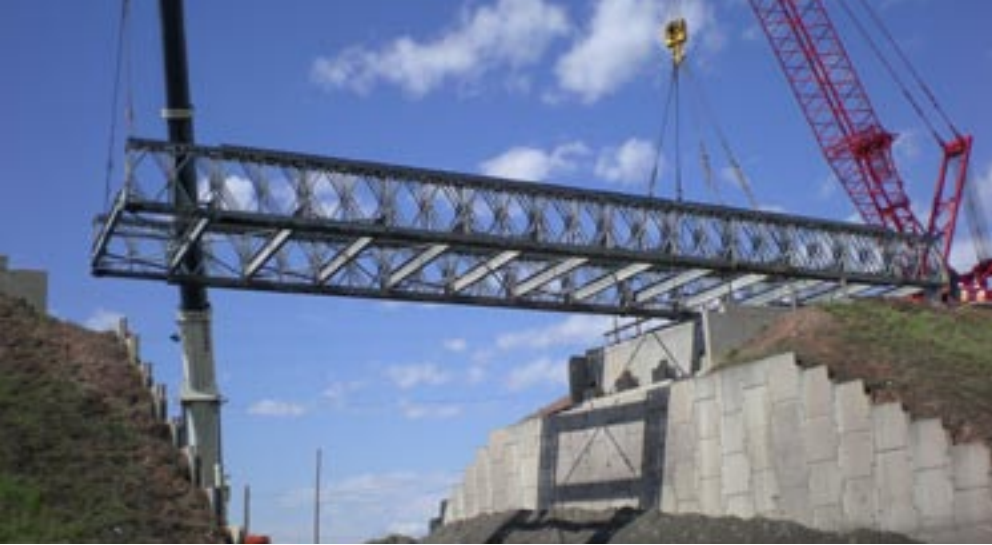
This 140-ft portable prefabricated modular steel truss bridge replaced the damaged span and allows for two lanes of traffic.
