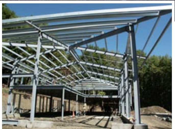
Steel and straw work hand in hand in Hakata House, a single-family residence in Upstate New York. Completed project, above; steel framing, below.
