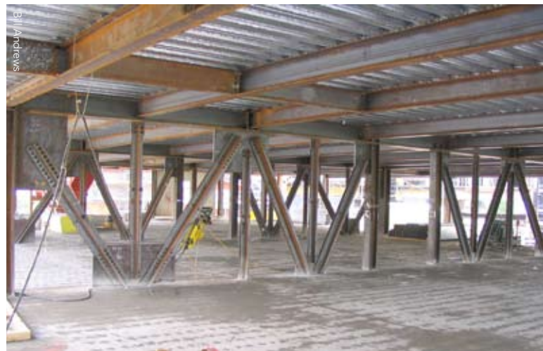
Story-height transfer trusses are enclosed in residential unit partition walls. Including a Vierendeel panel at midspan allows a corridor to pass through the truss.
