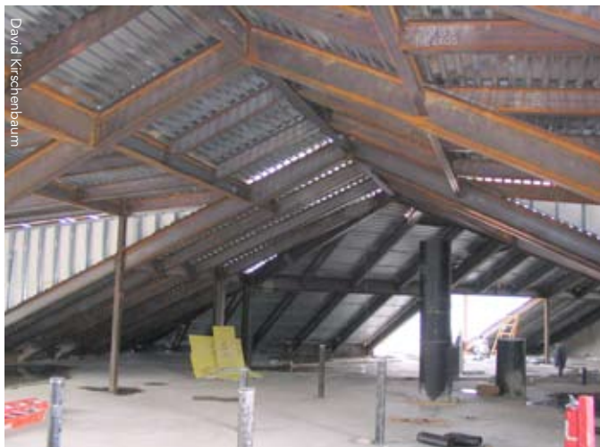
Steel framing sloped to varying pitches supports heavy snow drift loads while also providing usable attic space.
