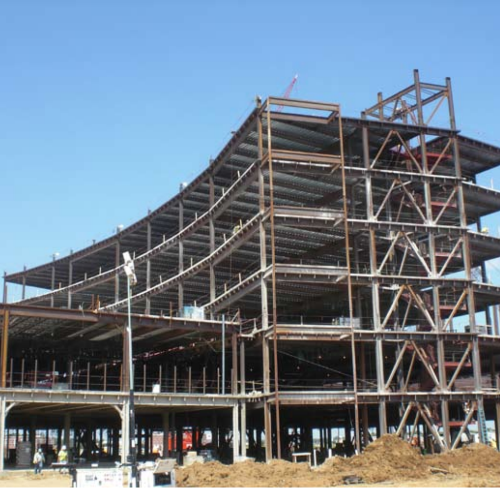
The architect's use of structural steel braced frames instead of concrete shear walls expedited the construction schedule.
