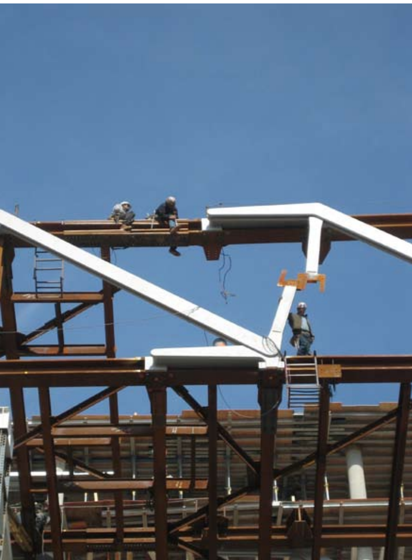
Below: The upper and lower web trusses, which provide the floor framing for levels 6 and 7, were joined on the north and south sides using prefabricated elements.
