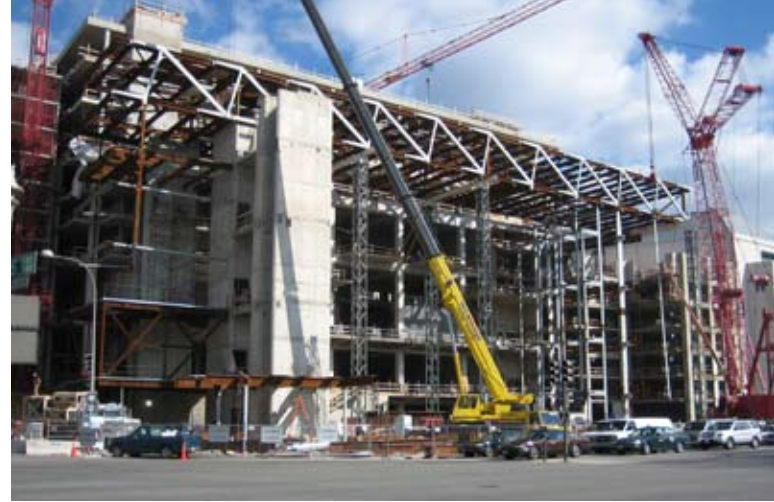
Erection of the 252-ft truss that spans the atrium. Its top and bottom chords are interconnected with prefabricated web trusses to create a long rectangular box. Photo: LERA
