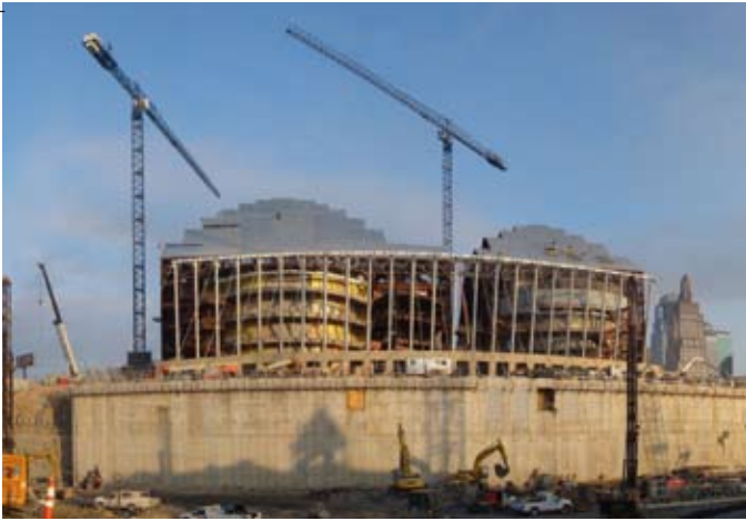
Instead of cables, slightly larger hot-rolled steel tension rods (visible in the foreground) are providing fire safety at the Kauffman Center for the Performing Arts, under construction in Kansas City, Mo., without the need to apply additional protective material.
