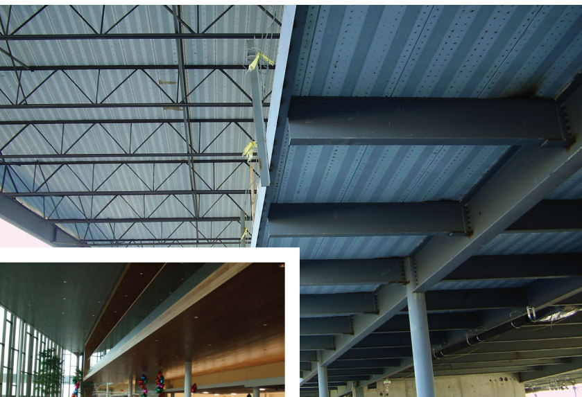
The dining area opens into a two-story open area and required a section of the second floor support to cantilever out from the columns.
