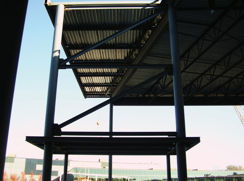
Left: This view of the dining room vestibule, from the inside looking out, shows the rigid frame on the second level. Note the offset in the pipe columns, by about half the pipe diameter, which was required to accommodate the difference in cladding between the upper and lower levels.
