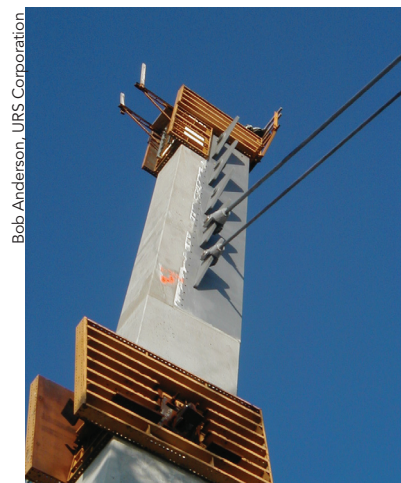
The pylon stay cable housing in place with the lower two back stays attached.
