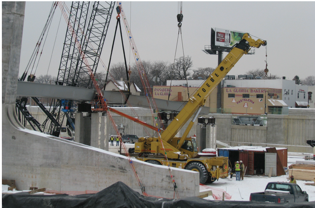
The complex erection sequence required the use of three falsework towers, which supported the west span until the cable stays were attached.
