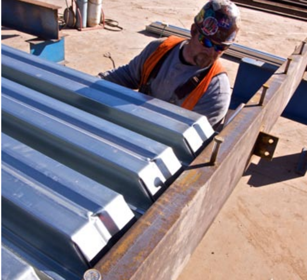
Factory closed ends of the Deep-Dek Composite floor panels rest on a dropped ledger angle shop-attached to composite channel beams.
