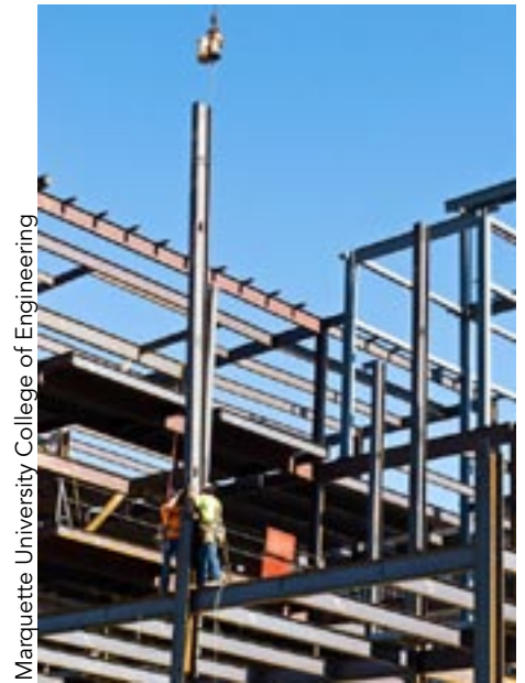
The steel frame of Marquette University's new five-story Discovery Learning Center provides the opportunity to use the whole building as an example of structural behavior.
