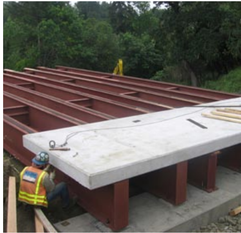
▲ Workers install the precast concrete panels that make up the deck of the temporary North Umpqua River detour bridge. Douglas County plans to reuse the deck panels and steel bridge rail at different sites after the permanent bridge is complete.
