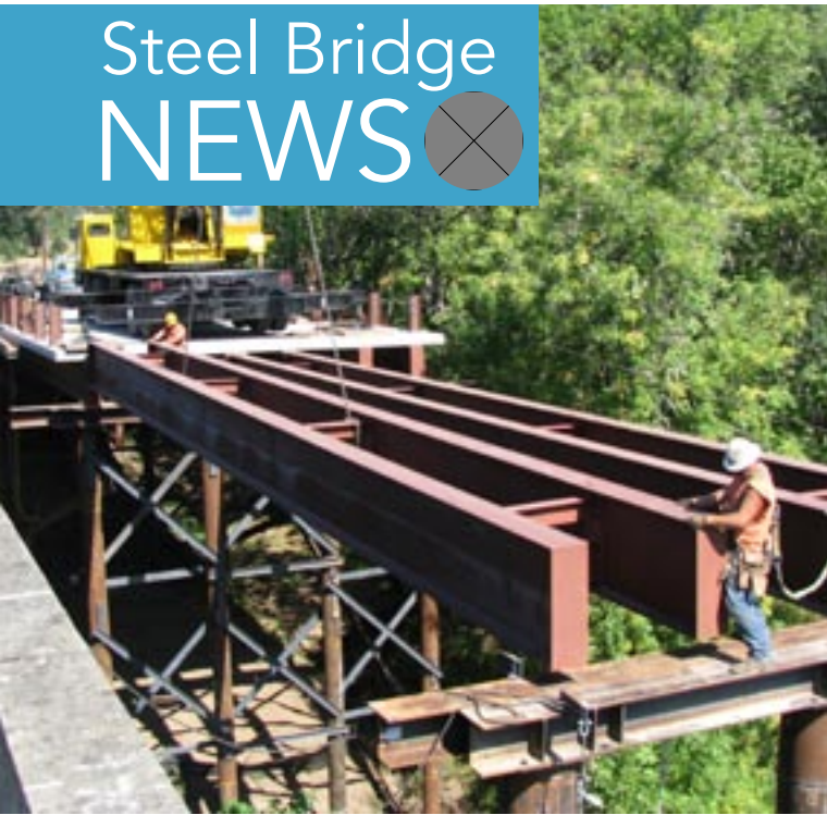
▲ The North Umpqua River detour bridge being constructed adjacent to the existing bridge. The steel girders for the 120-ft main span were salvaged and modified from a local bridge replacement.
