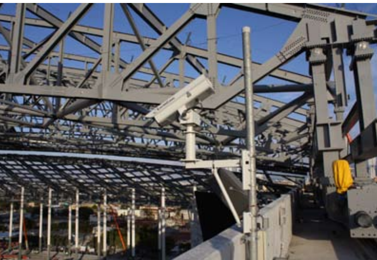
▲ The four-bar link on the south end of the lower roof section, showing three of the four pivot points.
