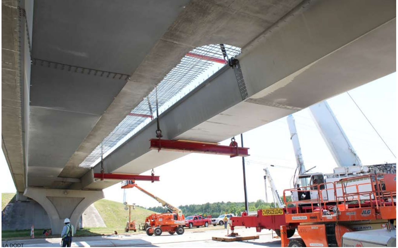
▲ The new section is put in place via a pair of cranes.
