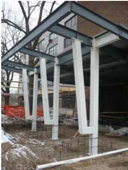
▲ Architecturally exposed structural steel for the canopy of an Indiana State University building.
