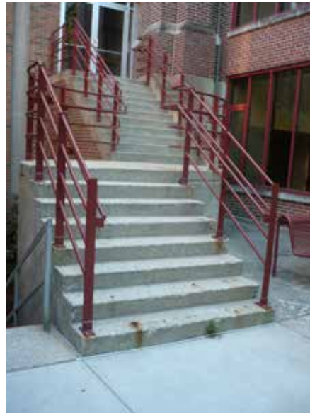
▲ An architectural metal handrail at a Rose-Hulman Institute of Technology—a typical miscellaneous metals project involving field measuring of steps following the concrete pour.
