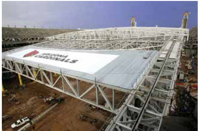
▲ The retractable roof of the University of Phoenix Stadium uses 402 tons of 12-in. square HSS.
