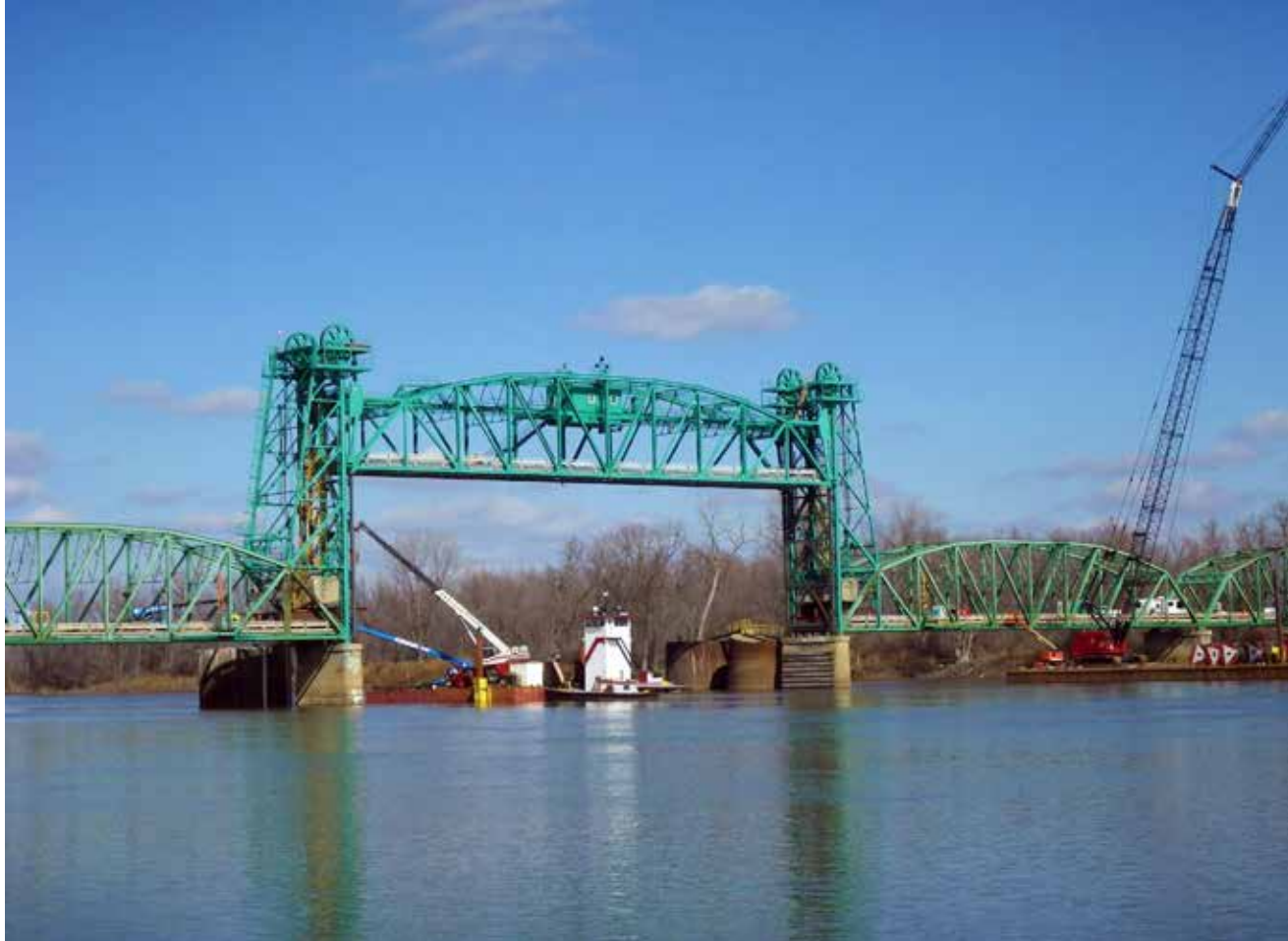
▲ The lift span was supported in the open position, thus allowing barge traffic to continue during the rehabilitation work.
