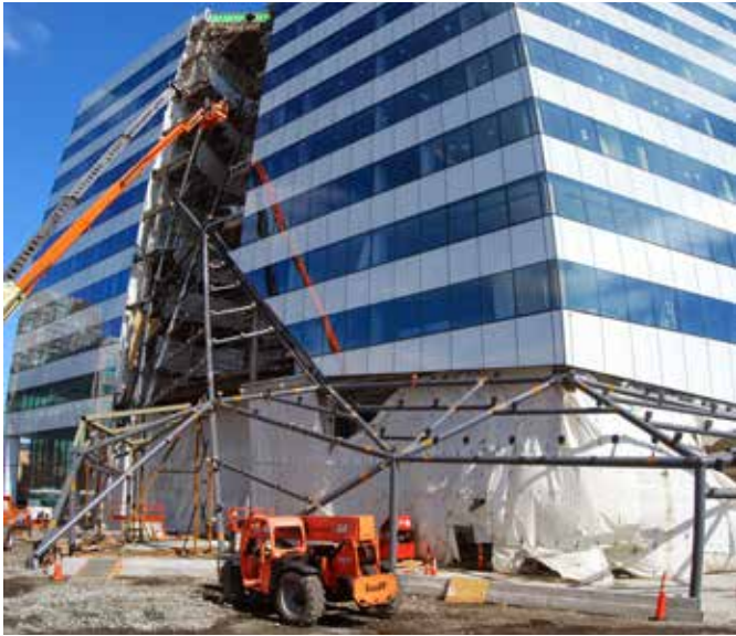
▲ Erection of the waterfall, which uses 100 tons of structural steel and spans the full height of the building.
