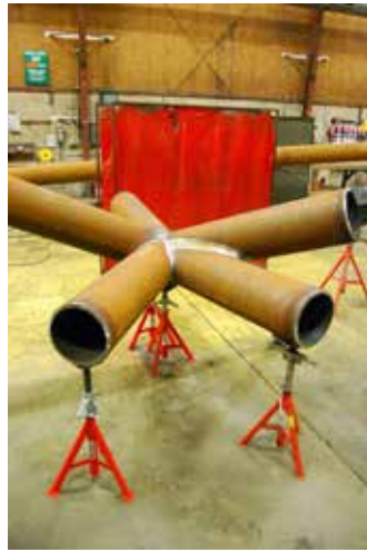
◀ An inside look at one of the waterfall node castings (left) and connecting a node to five round HSS (right). A combination of fillet and partial-penetration welds were used to complete the connections at each steel node.
