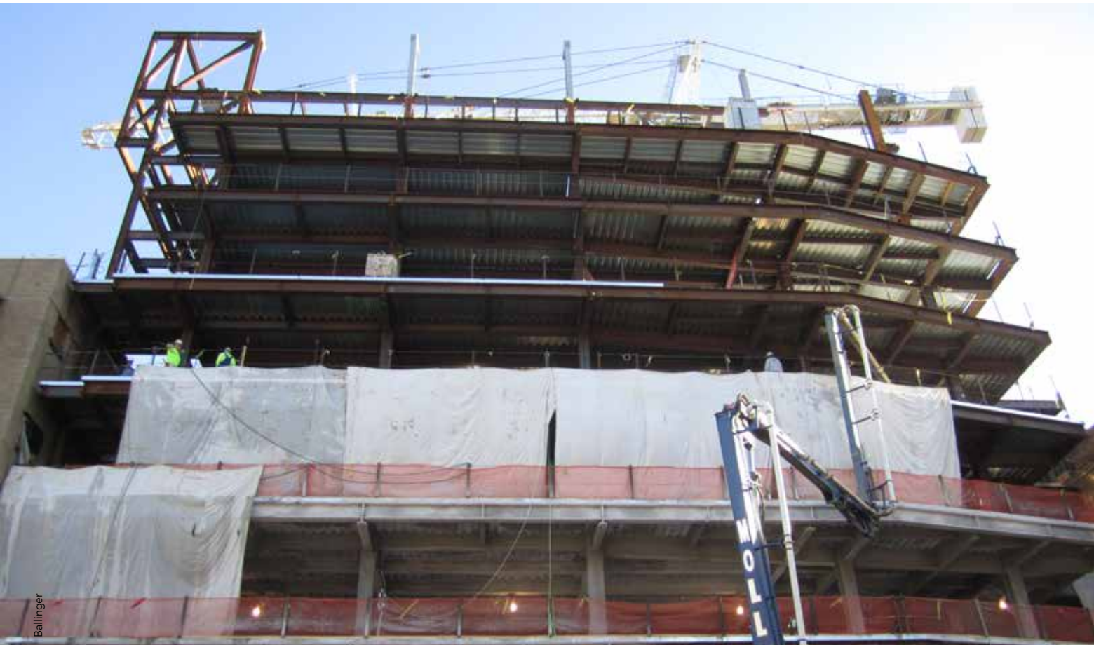
▼ Steel erection was performed by locating the tower crane within one of the elevator shafts.
