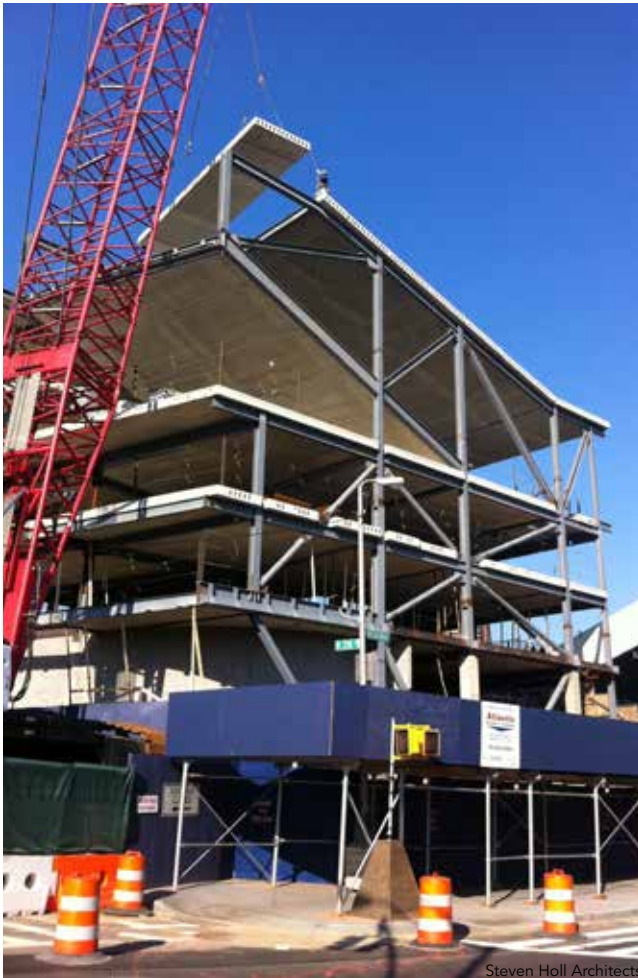
▲ The close proximity of the elevated subway tracks placed restrictions on the potential locations for crane placement, which influenced the erection sequencing of the framing.
