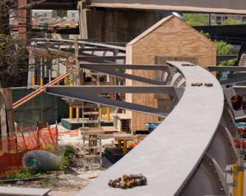
▲ Steel plate rib elements are connected to each side of the steel spine on 8-ft centers, tapering in depth from approximately 2 ft, 2 in. at the central spine to less than 5 in. at the outer deck edge.
