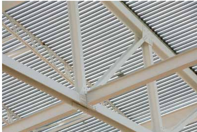
▲ Four different truss configurations are used for the roof. ▶ Steel framing for the seating.
