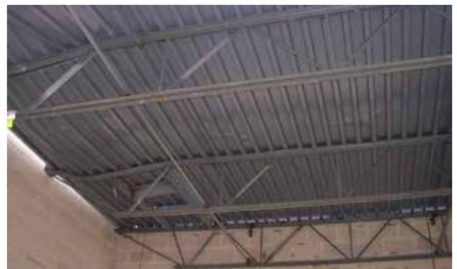
▼ Figure 6b. Separation between wall and roof deck.
