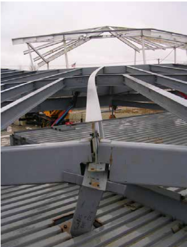
▲ Figure 3. The tension ring after initial failure.
