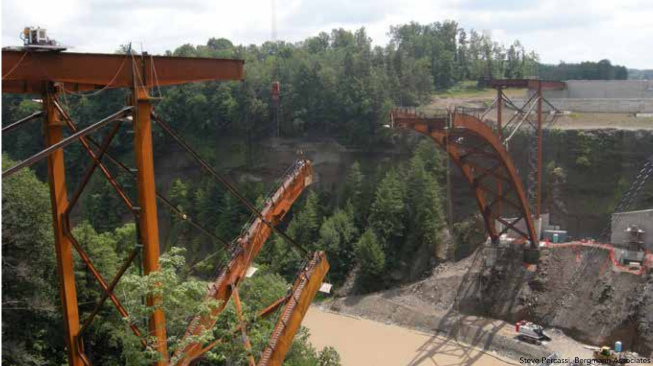
▲ The new specification provides long-needed guidance for contractors and their engineers who need to evaluate strength and stability during critical stages of erection.
