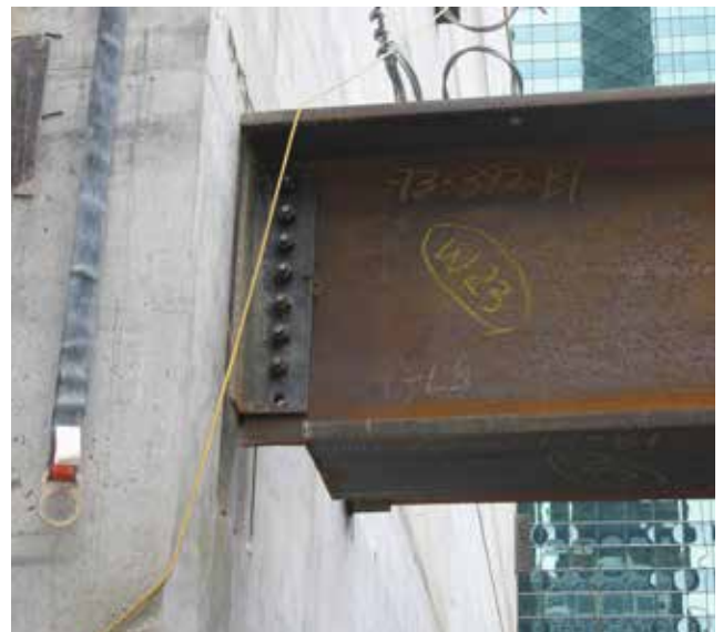
▼ Figure 2. Beam coped at the bottom flange.
