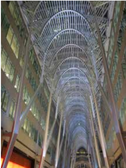
▲ BCE Place in Toronto (which predates any AESS standard) successfully used the principal of reducing levels of finish at the higher, less visible levels.
