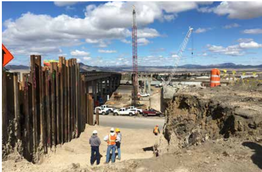
A critical part of the project sequencing was the requirement that the first new bridge be built during the first construction season.
