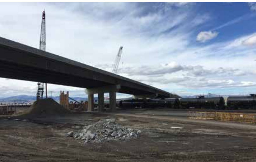
The chosen bridge span arrangement required three railroad tracks to be relocated in advance of construction.
