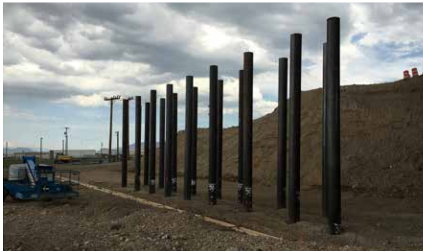
Crews had to deal with the area's relatively short seven-month construction season.
