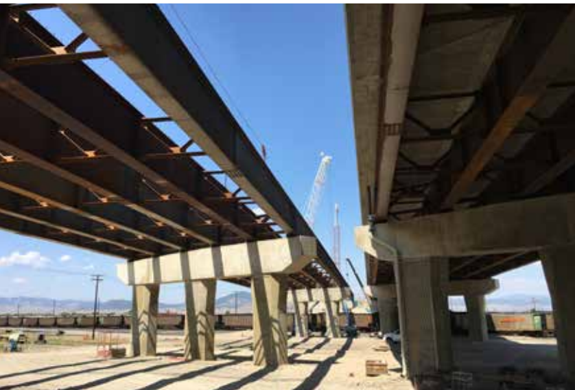
The team performed a comprehensive evaluation of the various bridge types and span arrangements and how they would impact the rail yard.
